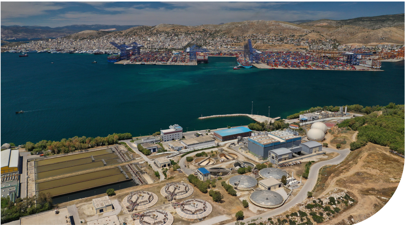
Aerial drone photo of latest technology sewage and sludge processing plant in small island of Psitalia or Psyttaleia, Piraeus, Attica, Greece (©Shutterstock, photo by Aerial-motion)
